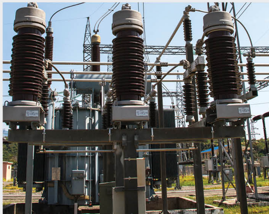
Measuring bay in the measurement point
