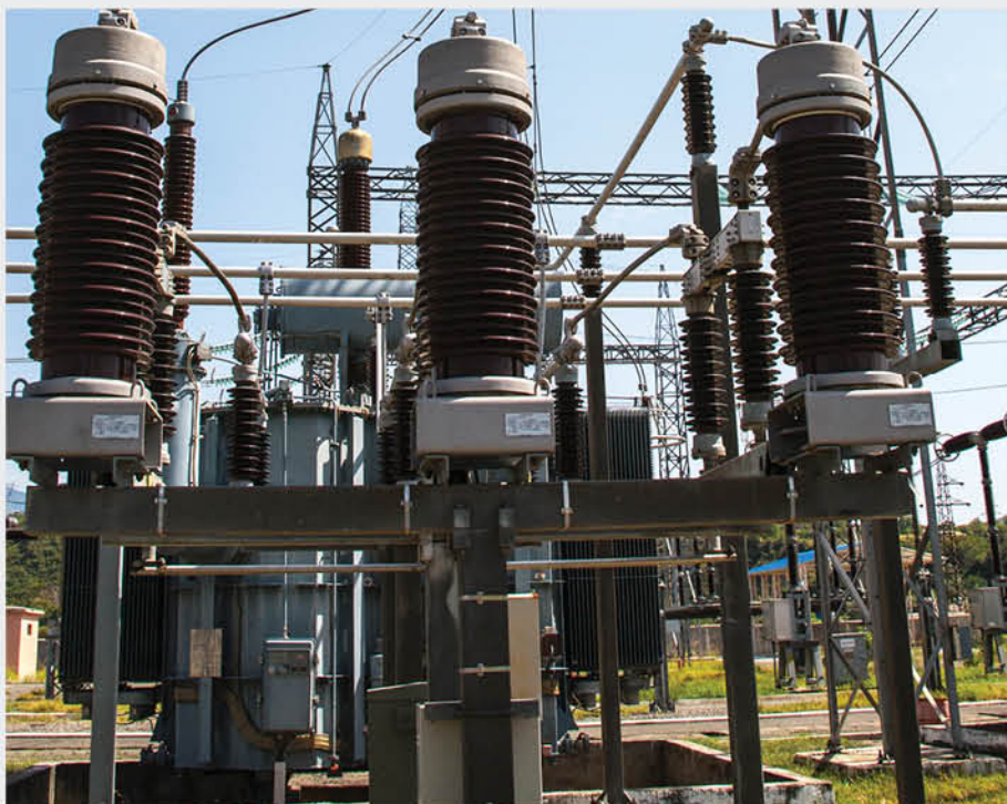
Measuring bay in the measurement point
